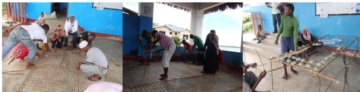
Figure 10: Trained community members assembling different parts to construct nursery cages. (Source: KMFRI 2014)
